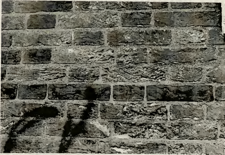
Figure 25 Spalling Caused by Brick Saturation Through Capillary Rise. 1998 Photograph by Author
